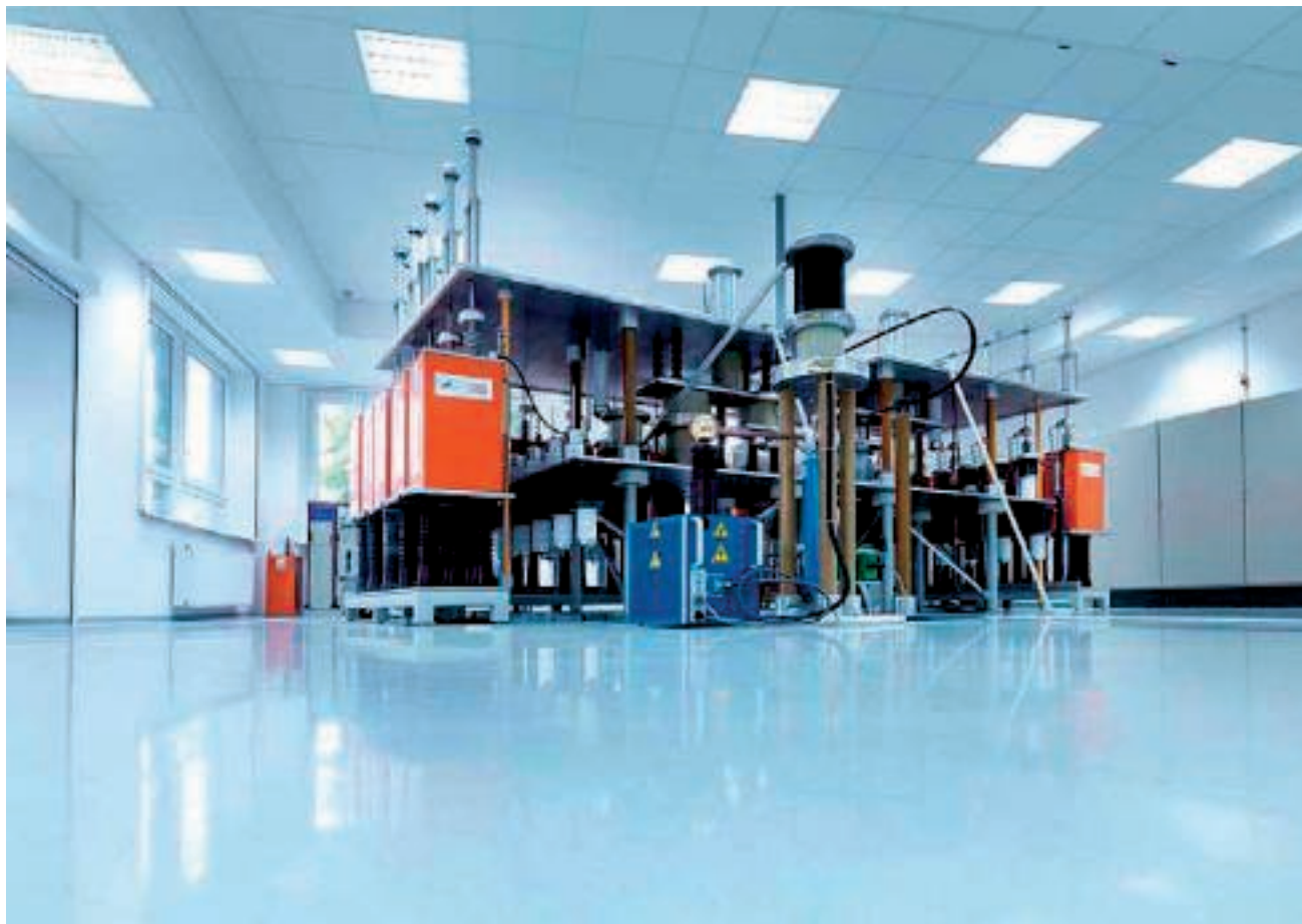
Lightning current generator
