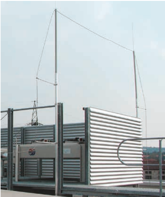
Figure 5.1.8.13 Isolated air-termination system with DEHNiso Combi
