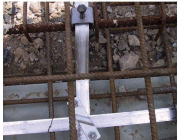
Figure 5.5.2.4 Foundation earth electrode in use
