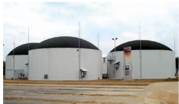
Figure 5.2.4.18 Protection of a biogas fermenter by means of a HVI Conductor
