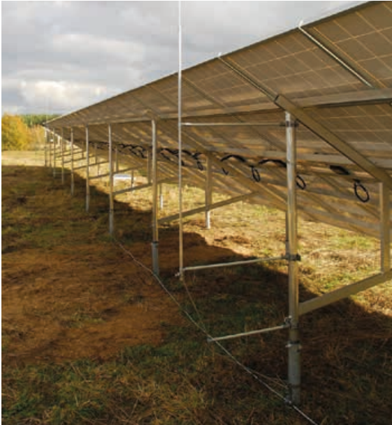
Figure 9.19.2 Lightning protection by means of DEHNiso spacers
