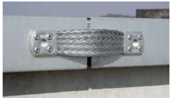
Figure 5.1.3.3 Bridging braid used for the roof parapet
