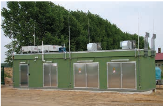
Figure 5.2.4.8 Protection of a biomethane plant by means of a HVI Conductor I
