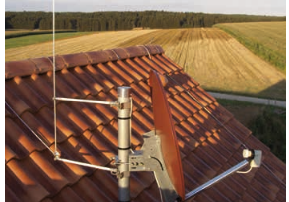
Figure 5.1.2.5 Antenna with air-termination rod and spacer
