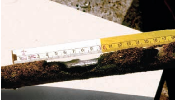
Figure 5.9.6 Corrosion of a galvanised earth rod after 7 years
