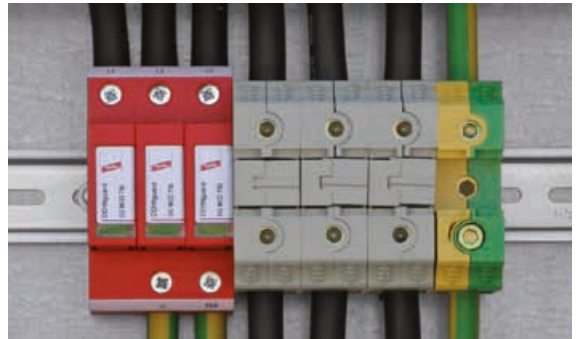
Figure 9.16.7 Protection of the stator side of the generator
