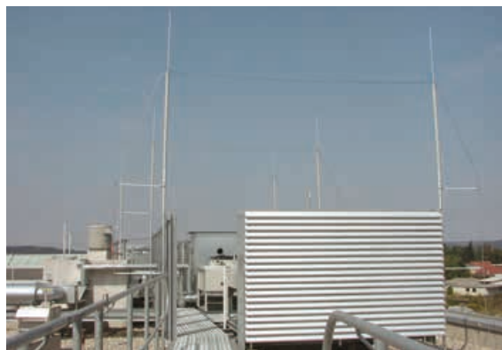
Figure 5.1.8.11 Isolated air-termination system with DEHNiso Combi
