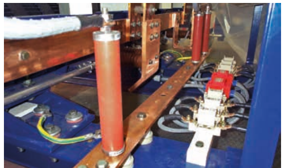
Figure 9.16.9 DEHNmid medium-voltage arresters installed in a transformer for wind turbines
