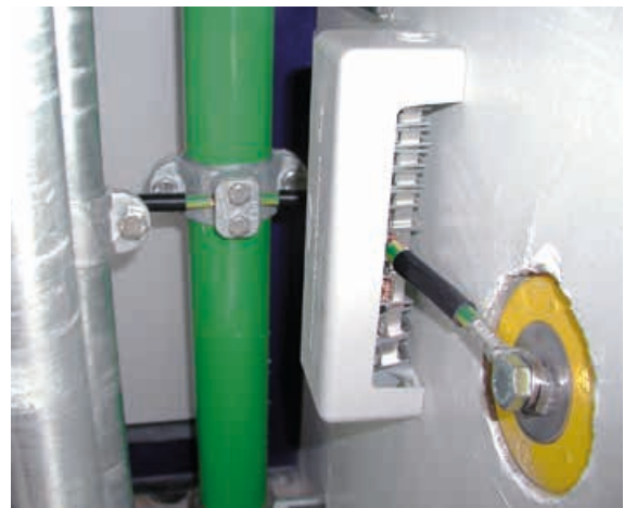
Figure 7.5.1.1 Connection of the EBB to the fixed earthing terminal
