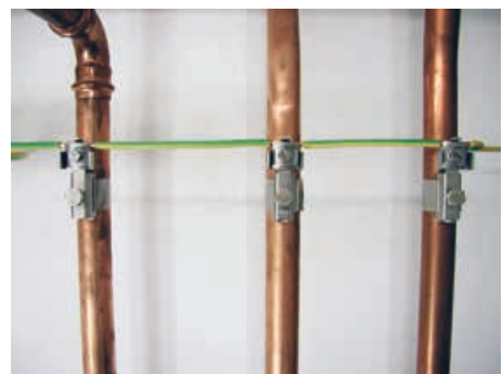
Figure 6.1.6 Through-wired equipotential bonding bar
